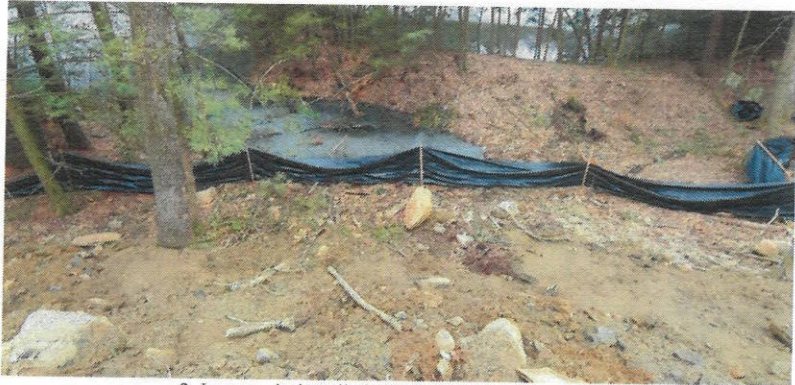
2. Improperly installed silt fence at edge of wetland
